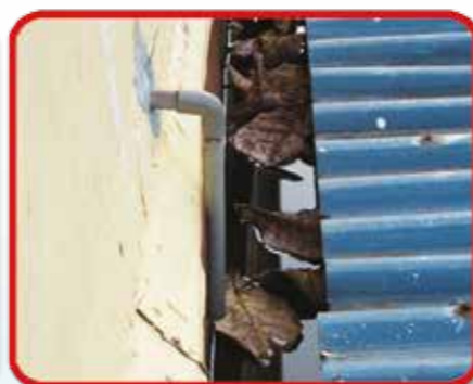
Clogged rain gutter
